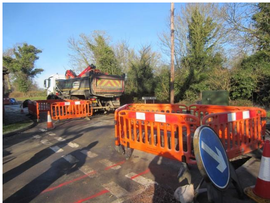
Keyham Water Pipes: see pages 3&4 for details
