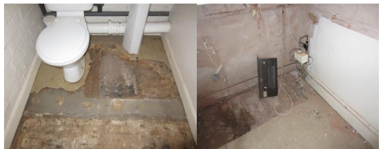
Rotten Floors: In Need of Repair!
