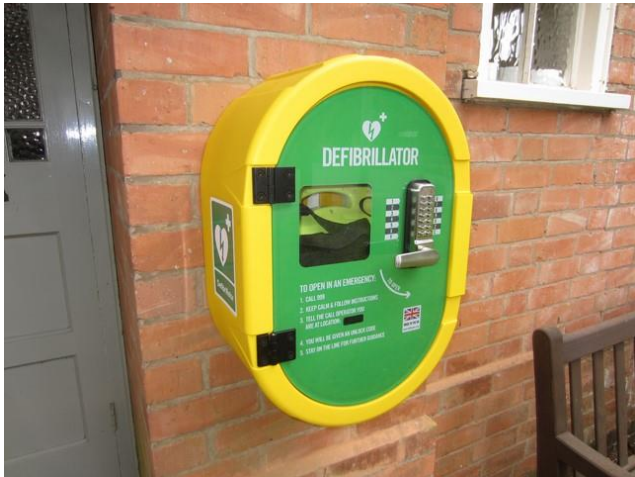
The Defibrillator is inside this cabinet at the Village Hall
